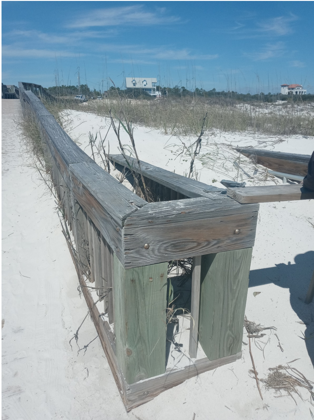
Figure 3: Mobile Street Boardwalk wheelchair ramp (right) completely overtaken by the dunes.
