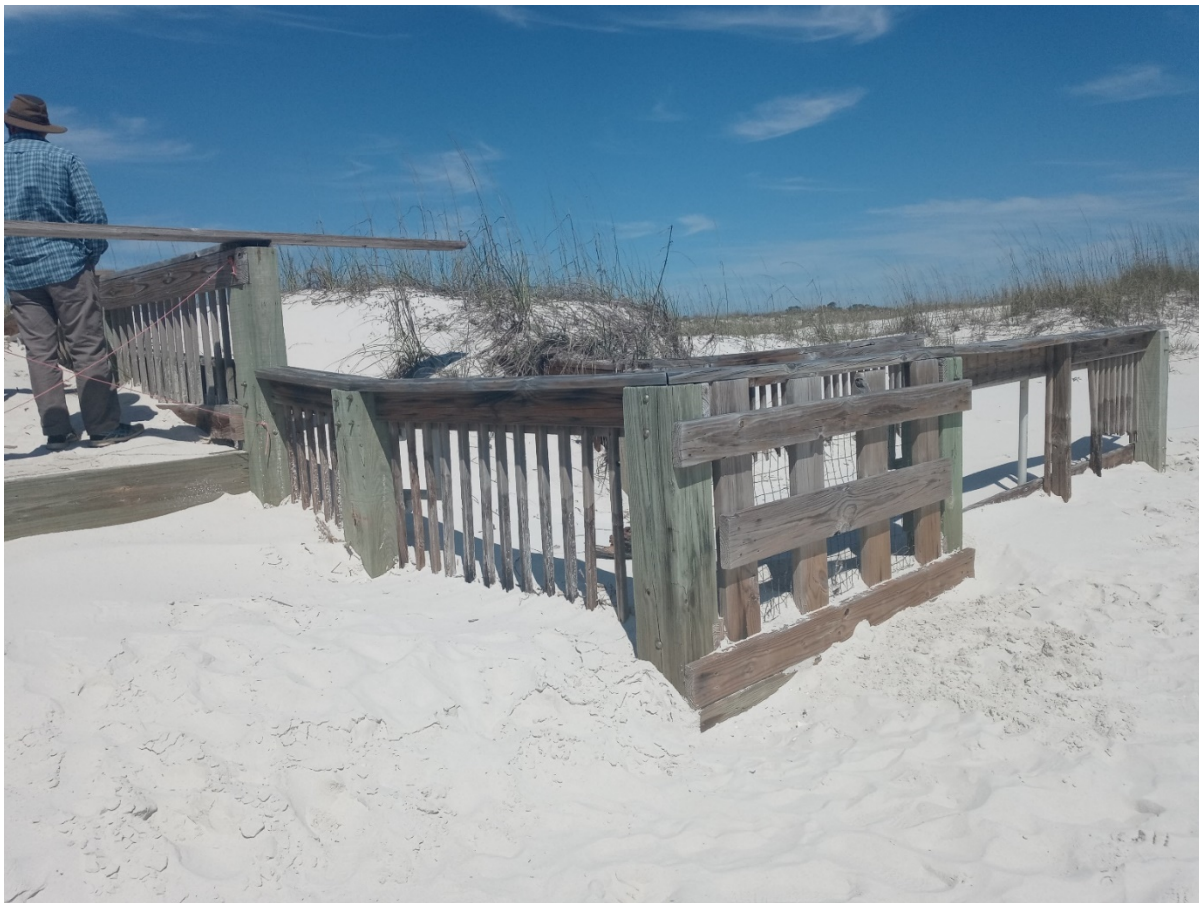
Figure 2: Mobile Street Boardwalk overtaken by sand.
